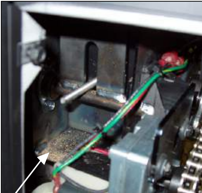
Possible pellet fines buildup area.
